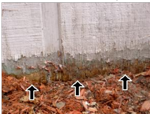
2.0 Picture 2 Siding deteriorated
