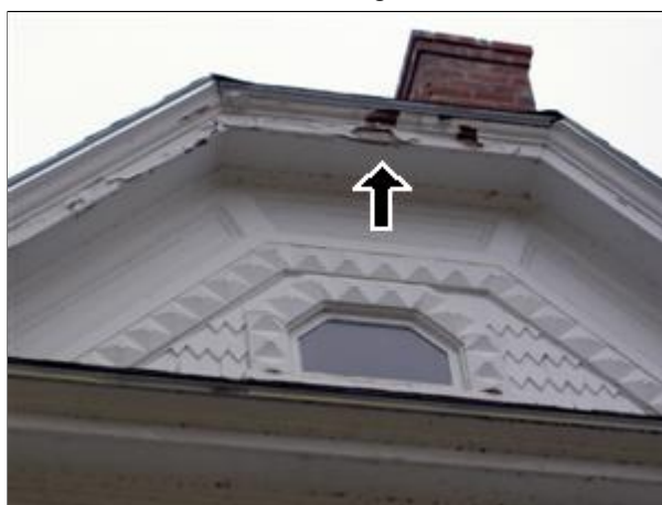
2.0 Picture 3 Exterior trim needs paint
