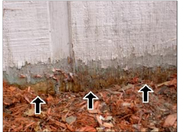
Item 2 - Picture 2 Siding deteriorated
