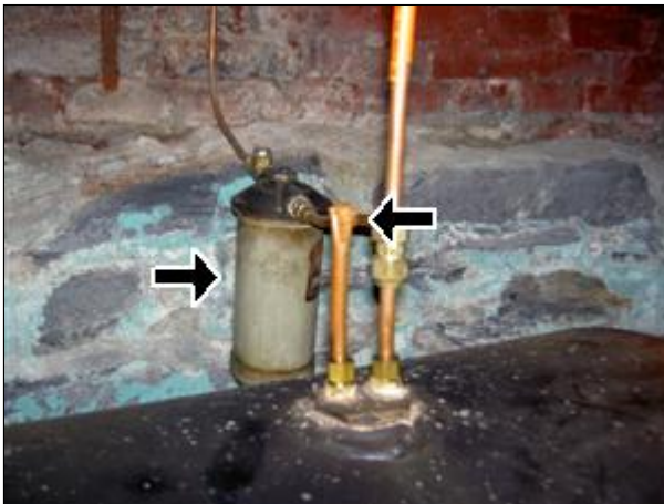
Item 20 - Picture 1 crimped oil tank outlet line
