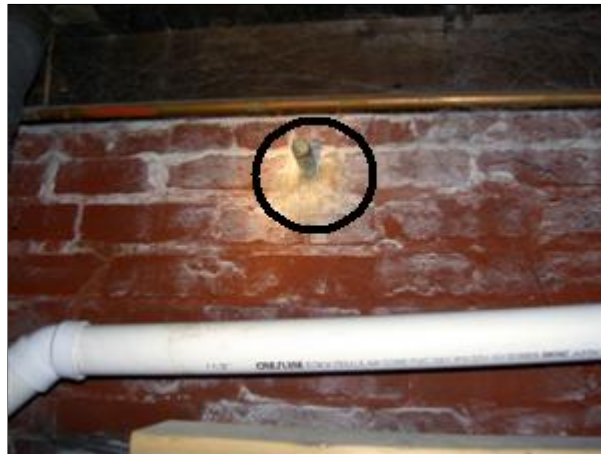
9.4 Picture 2 exposed pipe in the basement
