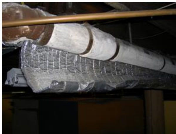
Item 26 - Picture 1 asbestos-like material
