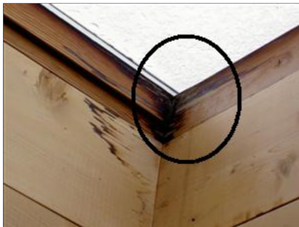
Item 1 - Picture 1 rotted wood
