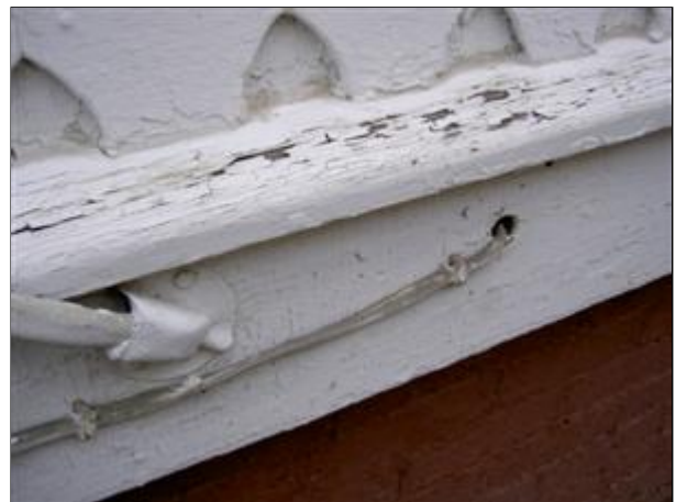
Item 2 - Picture 4 open holes
