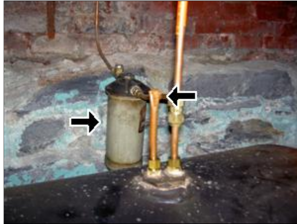
9.4 Picture 1 crimped oil tank outlet line
