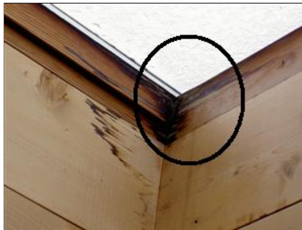
1.2 Picture 1 rotted wood
