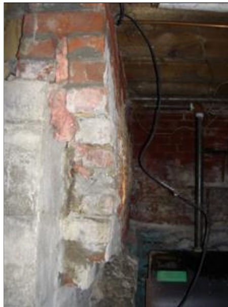
8.0 Picture 2 possible bow in cellar wall
