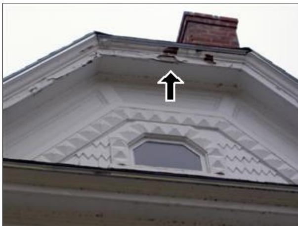
Item 2 - Picture 3 Exterior trim needs paint
