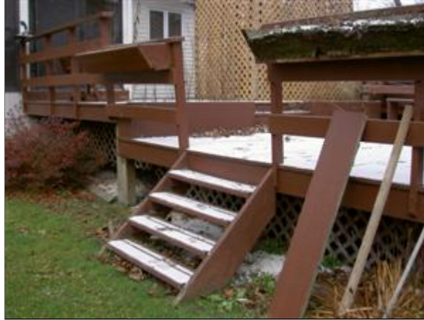
2.3 Picture 1 deck without handrail
