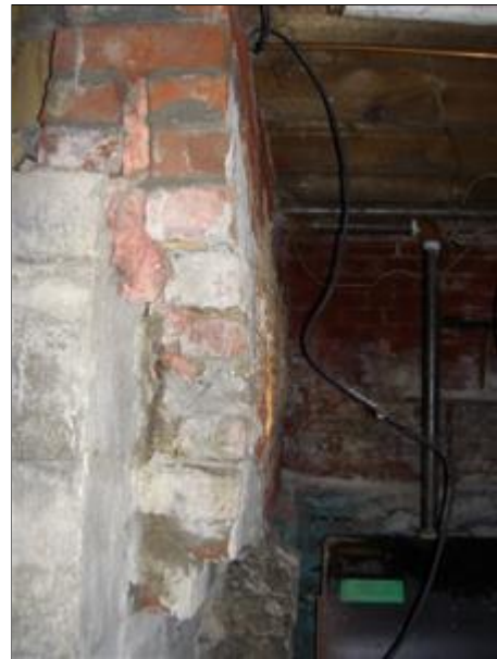
Item 16 - Picture 2 possible bow in cellar wall
