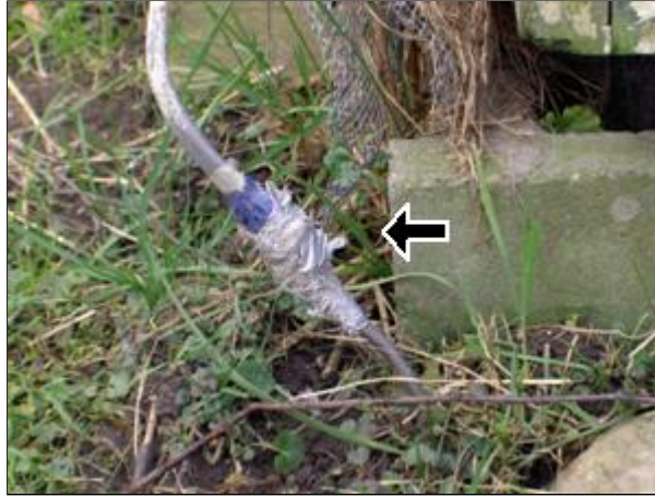
Item 21 - Picture 5 wire splice at garage
