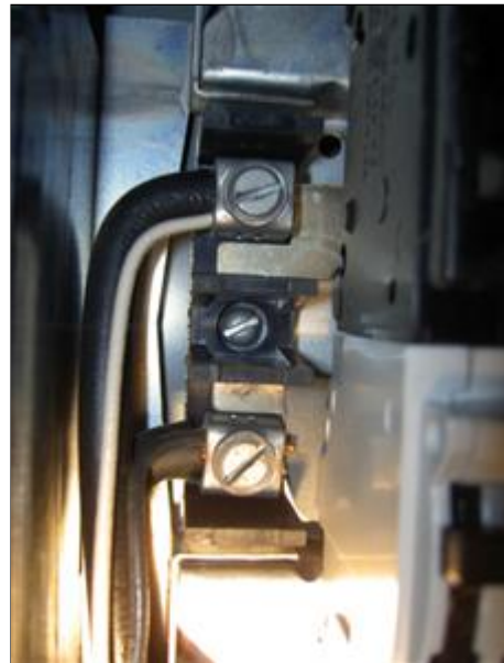
Item 21 - Picture 4 dryer tapped power
