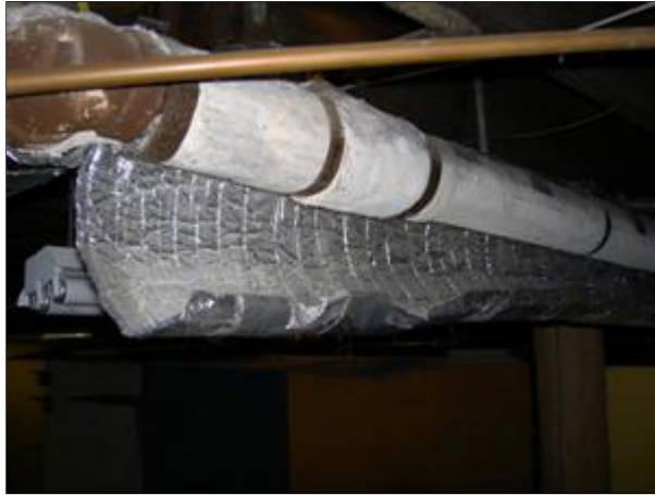
11.3 Picture 1 asbestos-like material
