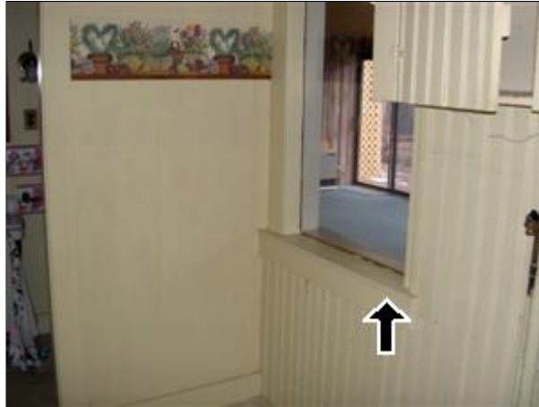
5.5 Picture 1 window not safety glass
