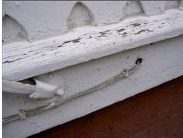
2.0 Picture 4 open holes
