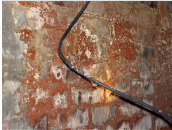
Item 16 - Picture 3 white effervescence on cellar wall
