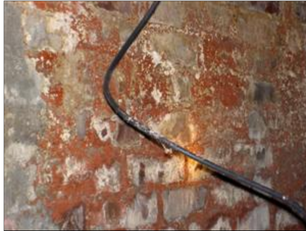
8.0 Picture 3 white effervescence on cellar wall
