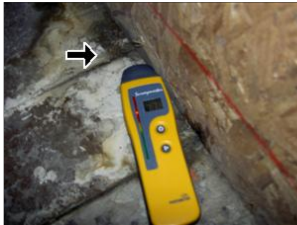
8.7 Picture 1 excessive moisture
