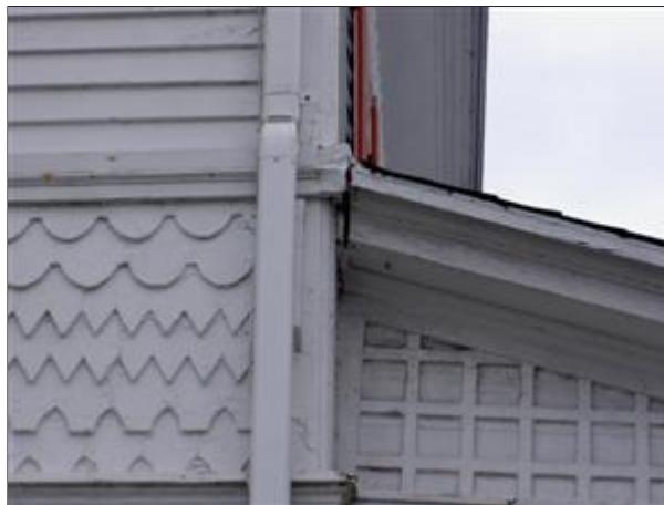
2.3 Picture 2 front porch settling
