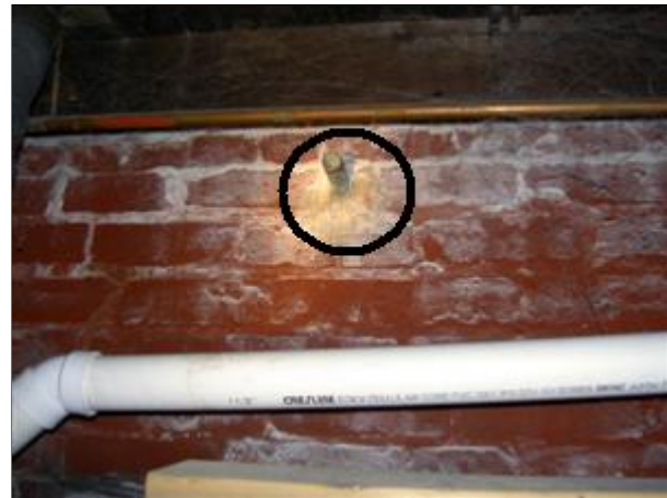
Item 20 - Picture 2 exposed pipe in the basement
