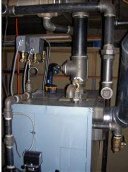
11.0 Picture 1 HB Smith boiler
