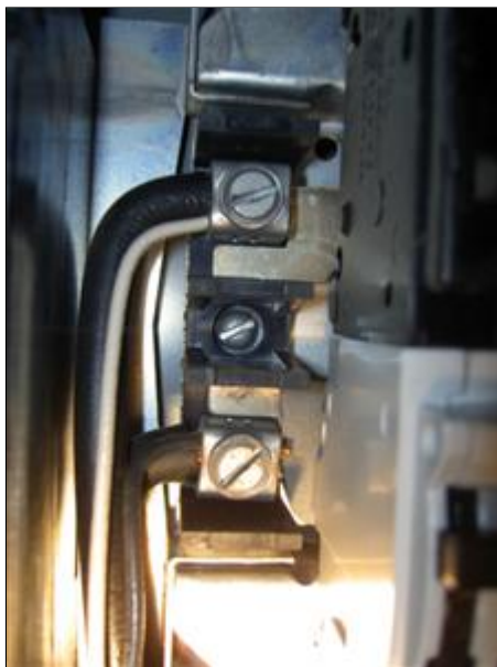
10.2 Picture 4 dryer tapped power
