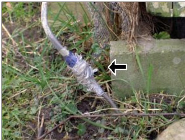
10.2 Picture 5 wire splice at garage
