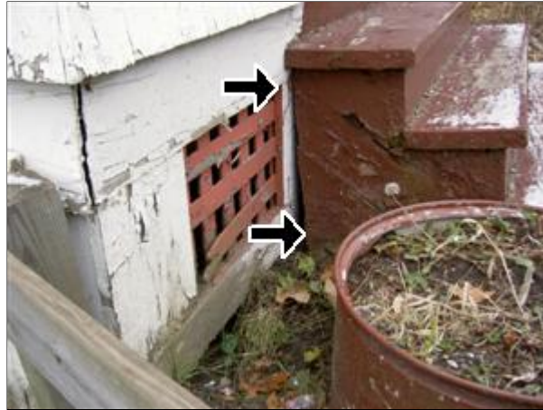
2.3 Picture 4 front step sagging
