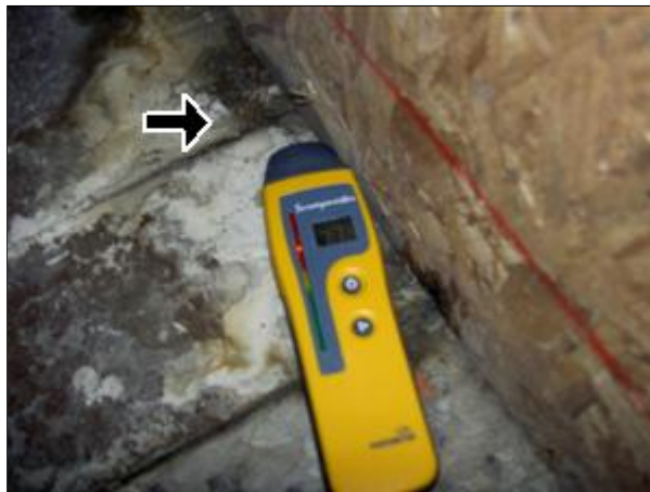
Item 17 - Picture 1 excessive moisture
